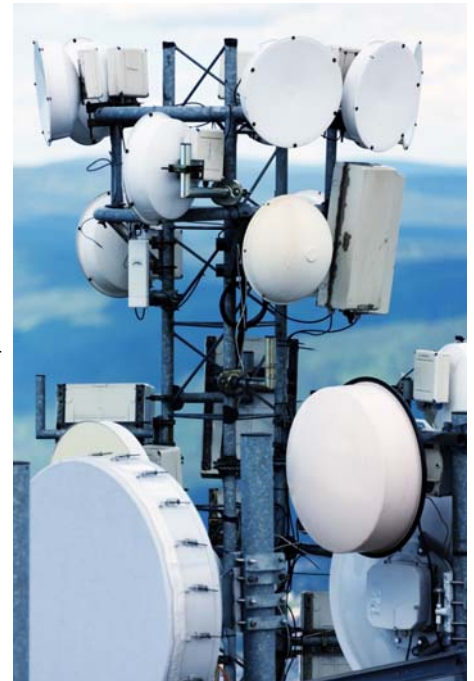
Microwave communications devices
