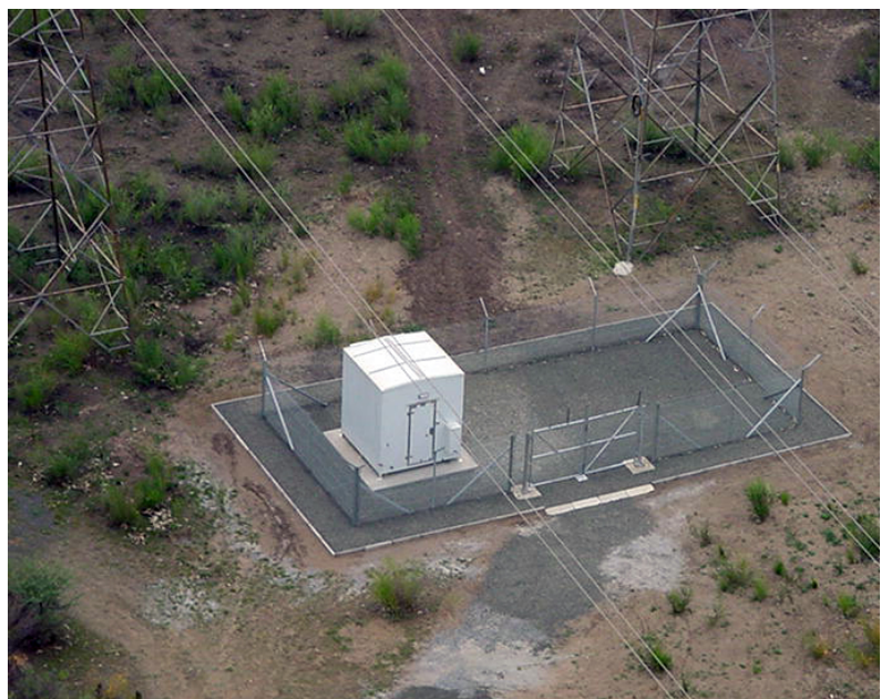
Figure 4: Typical Dual Container Repeater Site Located Beneath an HV Line (Image courtesy of Eskom & Broadband Infraco in South Africa)
