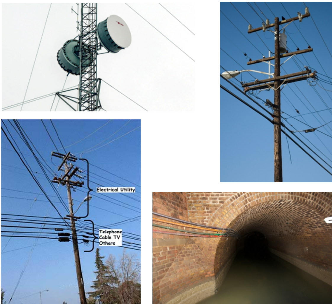
Figure 5: Images showing ICT Attachments to Utility Infrastructure
